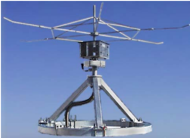
Shunt resistance installed at the top of tower
