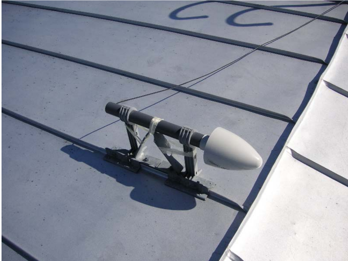
Figure 3: GPS-antenna at Ångström Laboratories roof
